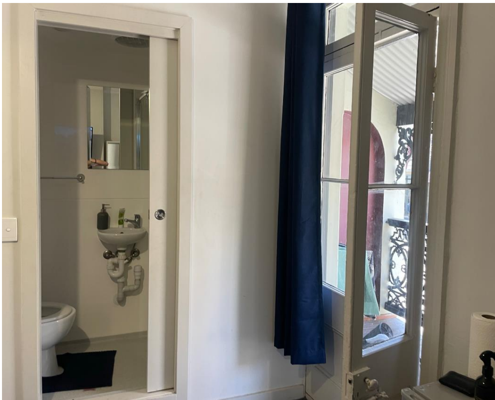
Figure 13: Room 3 with ensuite bathroom constructed without development consent
